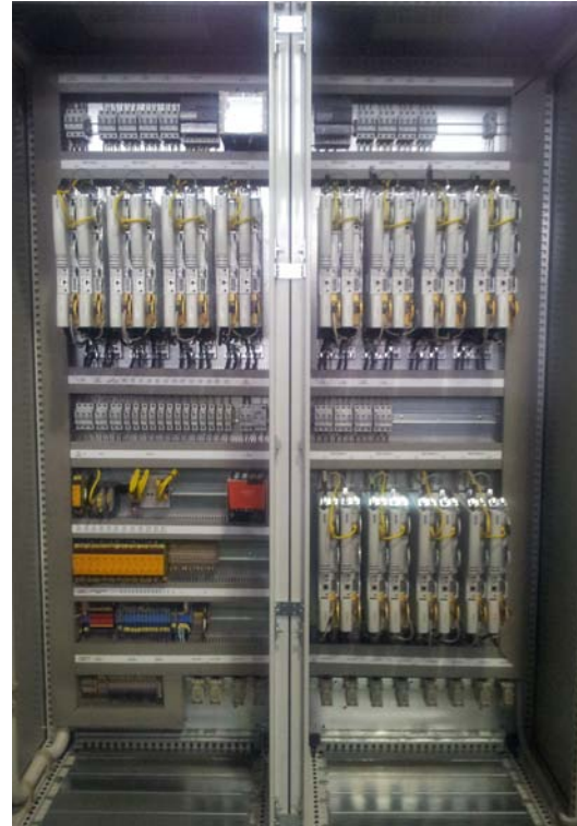
Converters and power supply points inside the cabinet
