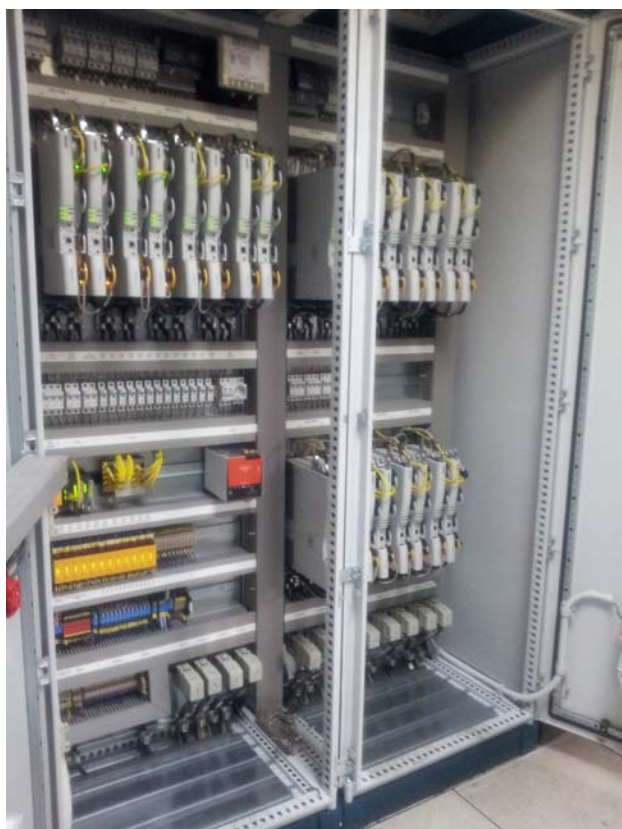
View of the power supplies and external out connectors arranged in the cabinet
